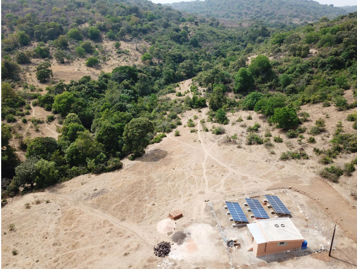
An off-grid solar installation in the town of Kouramangui, Guinea, implemented by Fondation Énergies pour le Monde (Fondem) in partnership with the Guinean Rural Electrification Agency (AGER) under the Petite Electricité Hybride en Guinée (PEHGUI) program. 109
